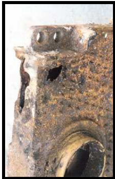
DAMAGED BOILER SECTION FROM SCALE
