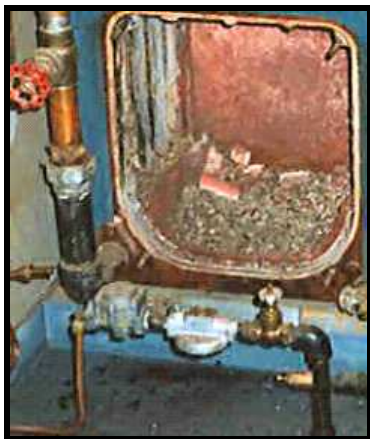
BOILER SOOT & HARD SLAG DEPOSITS PILOT STATION, ALASKA 2003
