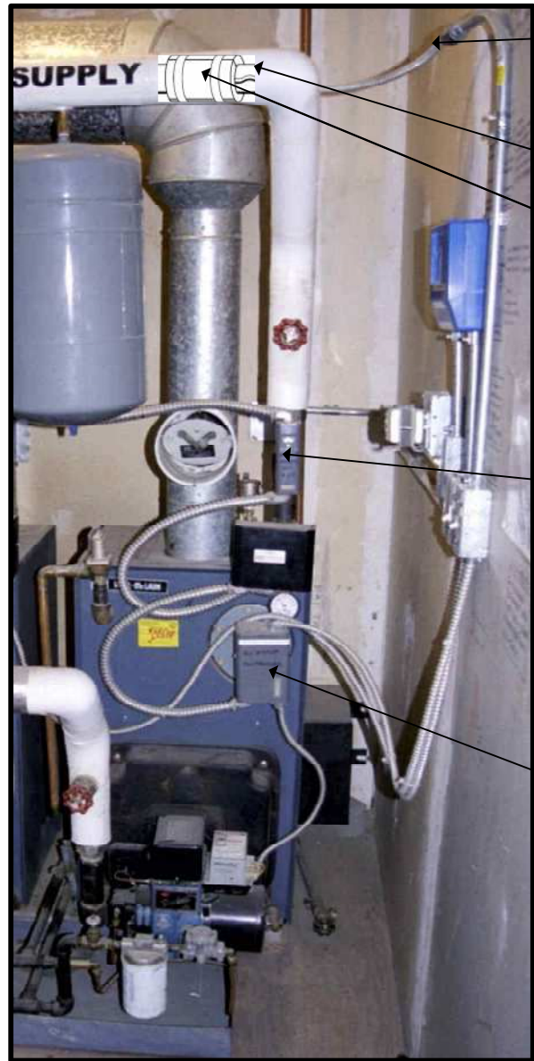
DUAL BOILERS – PILOT STATION NATIVE STORE For Demonstration Purpose Only For This Project Showing Proper Installation For A Commercial Installation, e.g. Conduit Above and
