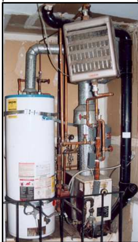
29 YEAR OLD BOILER, WITH OVERSIZED UNIT HEATER LIFETIME 1975-2004
