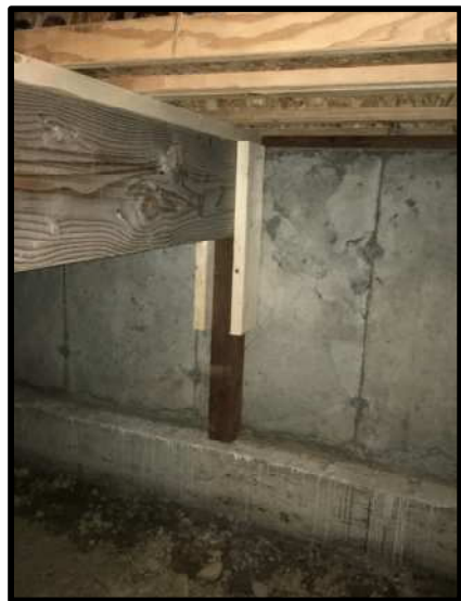
2 9-7/8" BC'S 4X12 BEAM 4X4 ALL WEATHER WOOD PIER CONCRETE FOUNDATION WALL & FOOTING
