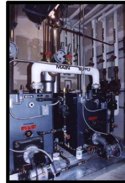
950,000 BTU Oil fired hydronic boilers with direct digital control installed by Jerry Nicholson in MarkAir's 22,000 sq ft Building in King Salmon Alaska
